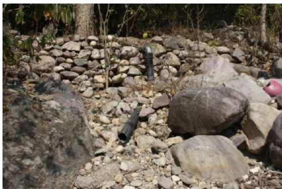
Sewage pipe draining out to beach
