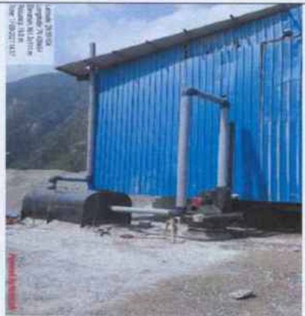
Dust extraction system
