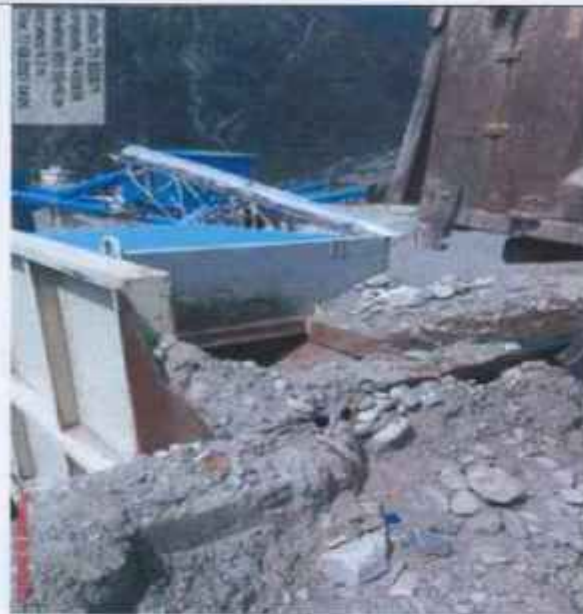
Covered process area
